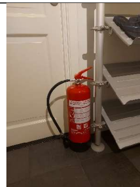
Fire extinguisher in the hallway on the first floor.
